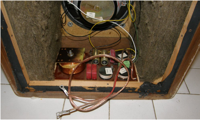
Replacement of the cables going to the terminal block. HP wires are large enough not to require changing.
